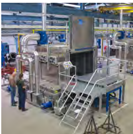
Gas heated tanks with work platform
