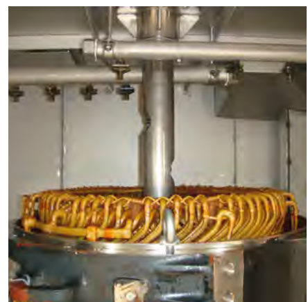
Lance system for internal cleaning of the stators
